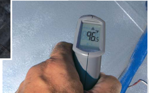
VFI-540 Aluminum Rubber Roof Membrane temperature
